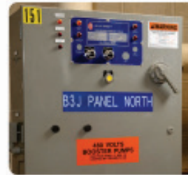
Control Panel & Electrical Panel Labels
